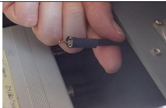
Figure 17: cable as found.
